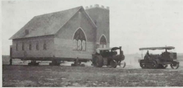
St. John's Lutheran Church was one of several churches moved from the original town site. Congregation members held church while the church was in transit.
